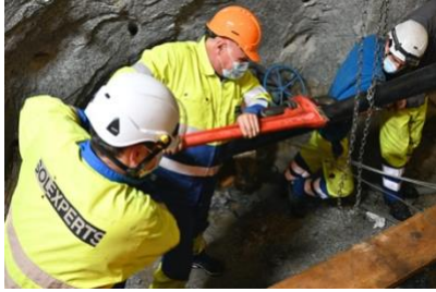
Installation of packers to isolate the stimulation intervals in borehole ST2 at the Bedretto Laboratory of ETH Zurich. The work was carried out under the direction of Geo-Energie Suisse.
