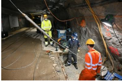
Installation of a seismometer chain in borehole ST1 to monitor the stimulations in borehole ST2, at the Bedretto Laboratory of ETH Zurich. The work was carried out under the direction of Geo-Energie Suisse.
