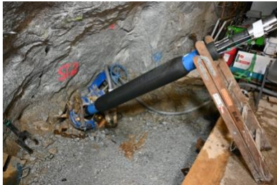
Installation of packers to isolate the stimulation intervals in borehole ST2 at the Bedretto Laboratory of ETH Zurich. The work was carried out under the direction of Geo-Energie Suisse.
