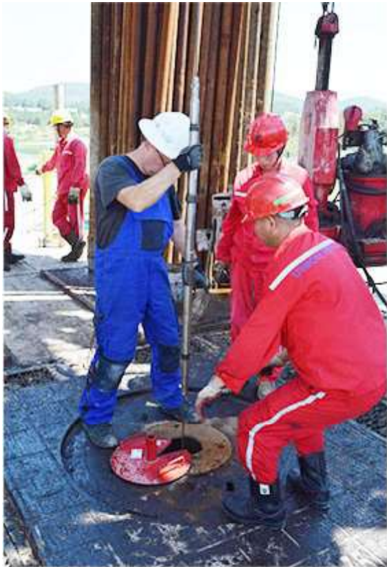
Installation of the geophone chain into the well PX-2 (view from the rig floor).
