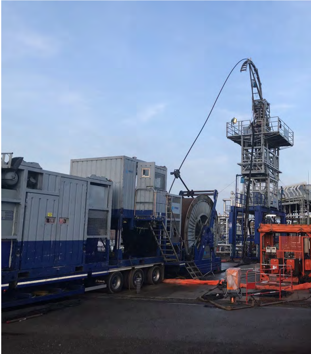
Figure 22: Setup of the coiled tubing in the wellhead of GPK-4, from the coiled tubing unit on the left to the coiled tubing frame on the right.
