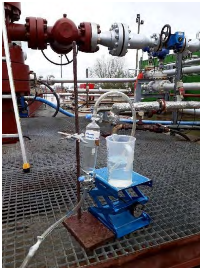
Figure 17: Gas sampling at GPK-3 wellhead degasser. April 2019
