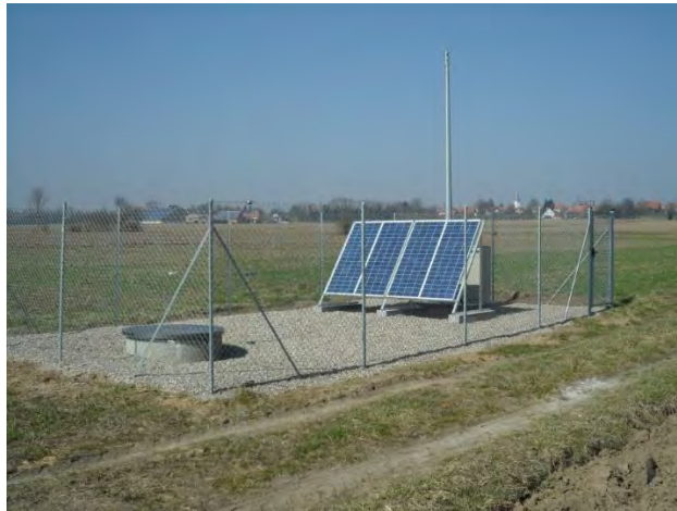
Figure 11. View of a permanent station from the Rittershoffen network.
