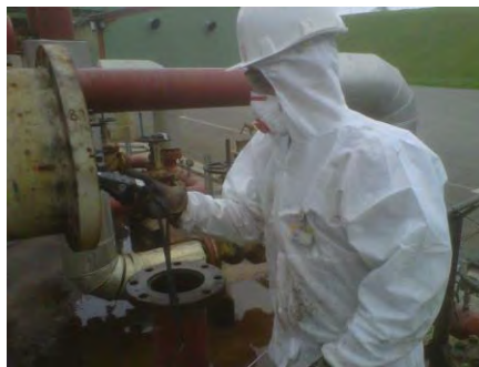
Figure 9. Example of individual protective equipment worn for the opening of a heat exchanger.
