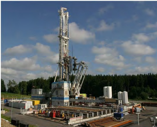
Figure 24. (Left) UDDGP concept showing theoretical well intersection with the targeted fault. (Right) The Anger's Sohne Innovating with hydraulic pipe handling system use to drill both UDDGP wells (Ledingham et al., 2019 and Law et al., 2019).
