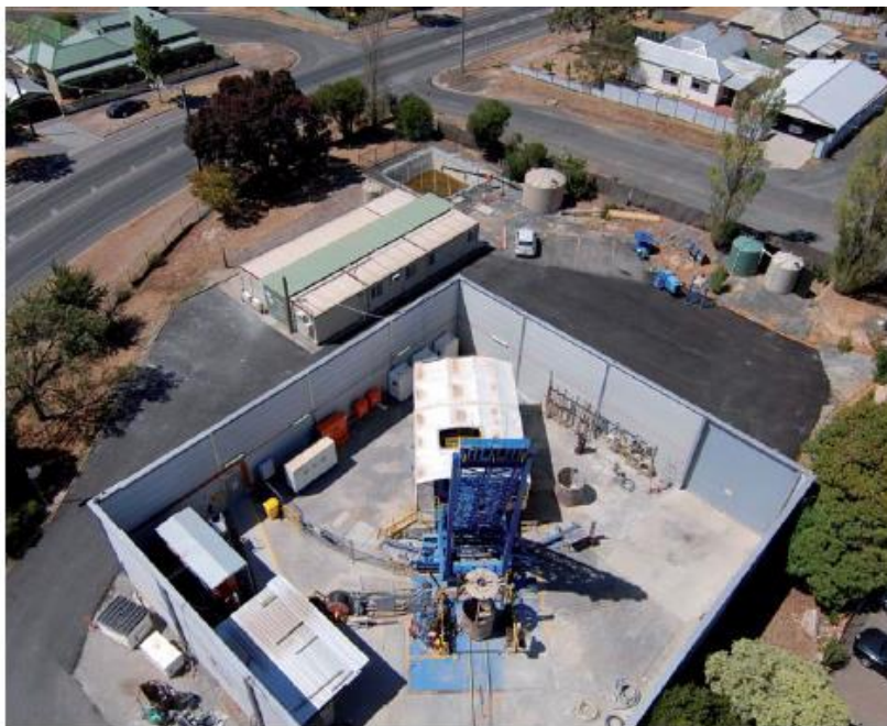
Fig. 18 View of the anti-noise barriers installed on a urban working site (DIIS , 2011)
