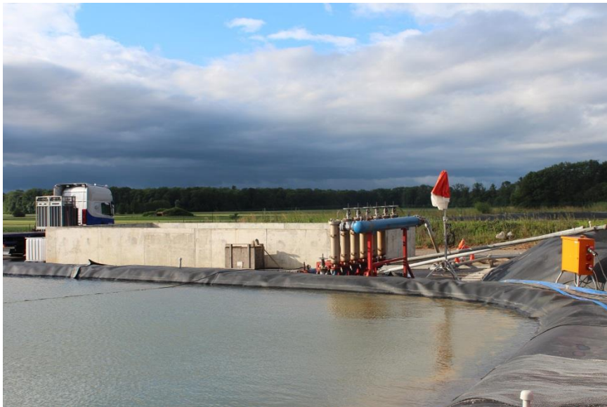
Fig. 19 Basin for brine storage during the chemical stimulation at the Rittershoffen geothermal site (France). ©és
