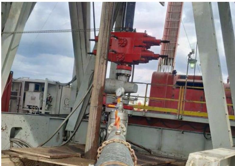
Figure 1: Wellhead with pipeline for stimulation (© EnBW)
