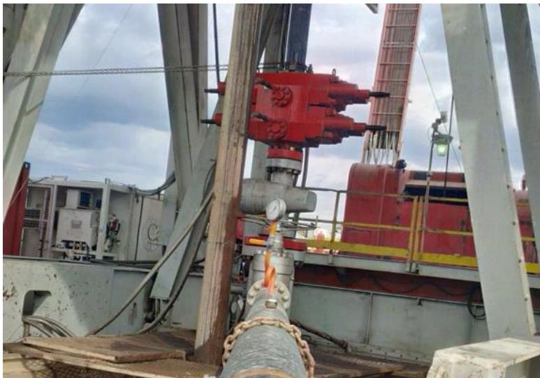
Fig. 1: Wellhead with pipeline for stimulation. © EnBW
