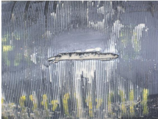
Figure 9: Example of damaged inflatable packer in Triemli.
